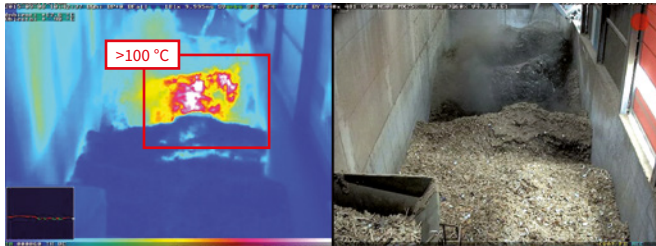
Thermal Radiometry (TR) automatically generates an alarm if the temperature exceeds or falls below the pre-defined temperature range.
